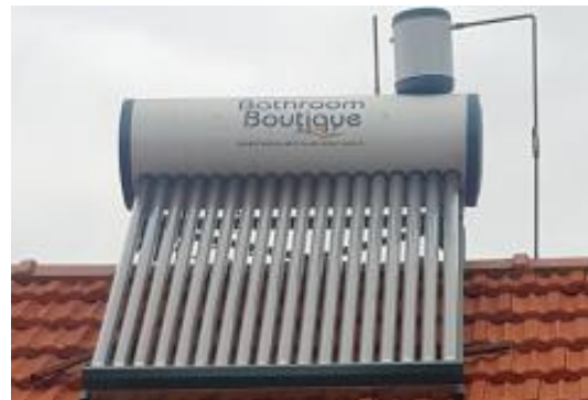
FIGURE 10. A TYPICAL SOLAR SIPHON SYSTEM COMBINING A COLLECTOR WITH A TANK, HERE INSTALLED ON A MSF BUILDING IN ZIMBABWE.
