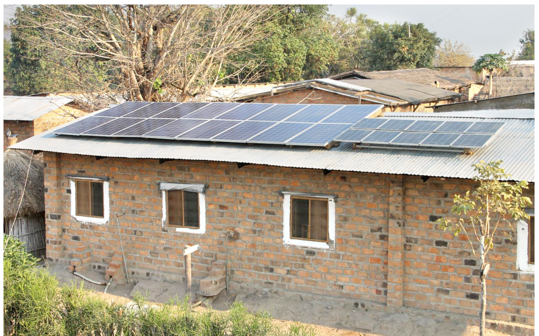
Solar installation in Shamwana, DRC
